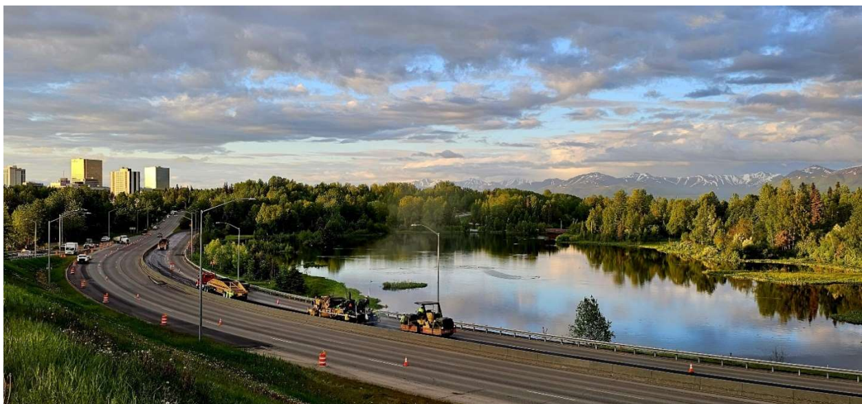
Minnesota Drive: Tudor to 15 th Ave Pavement Preservation Paving operation in Anchorage (West Chester Lagoon), Summer 2023.
