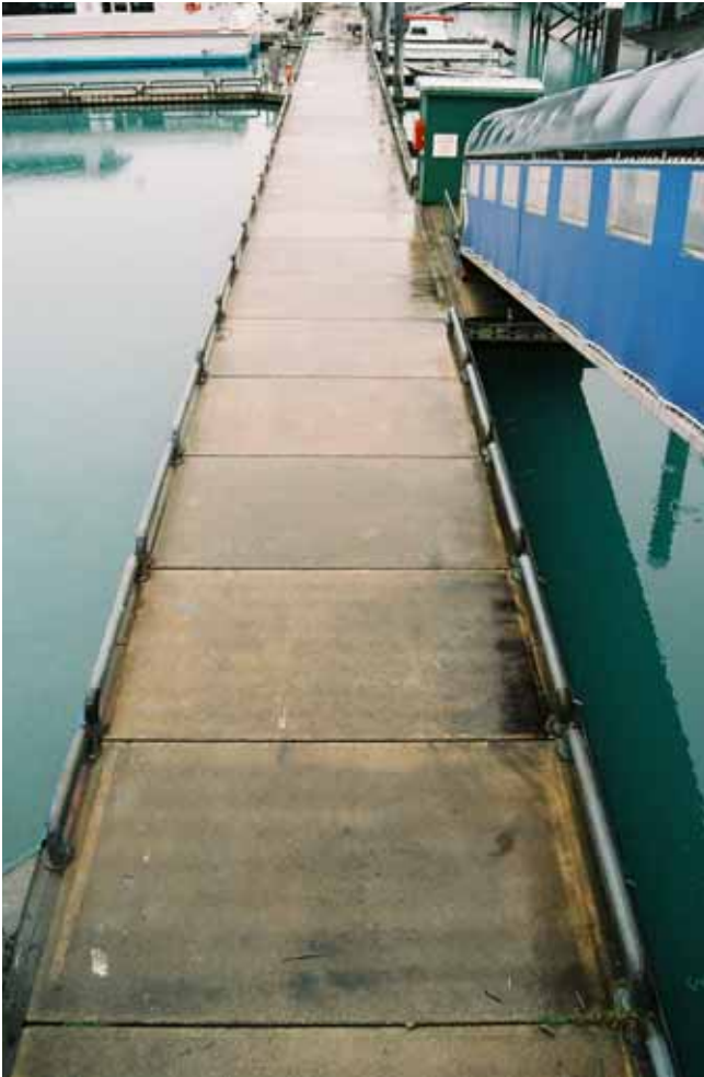
The longevity of concrete floating docks has greatly improved since the 1970s, due to better manufacturing technology.
