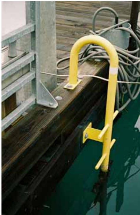
Safety ladder, installed according to Transpac Marinas mechanical drawing, in Valdez Harbor, Alaska.
