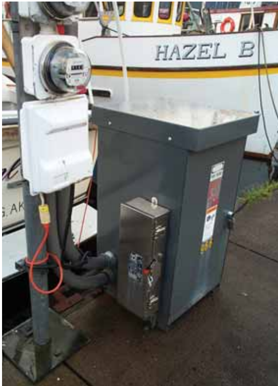
Marine transformer (note non-approved cord).
