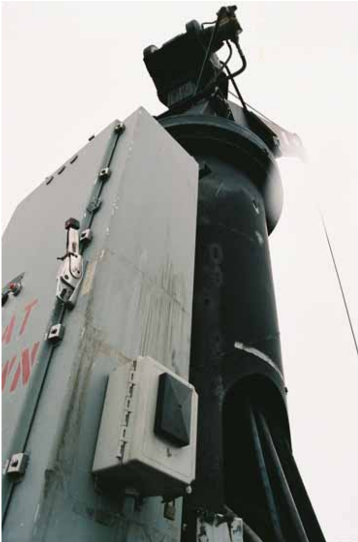
The access card reader box, using ALX technology, on a crane in Valdez Harbor, Alaska. This system provides a complete record of users and hours of operation.
