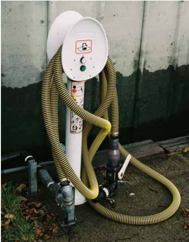
Sewage pumpout station in an Alaska harbor. The Clean Water Act prohibits dumping raw sewage in U.S. waters.
